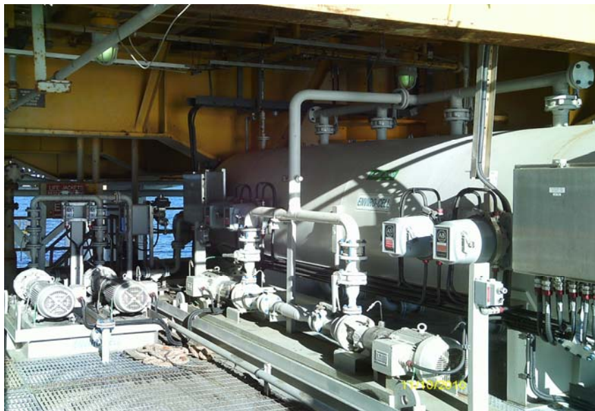
Figure 2: Enviro-Cell unit installed on the platform.
